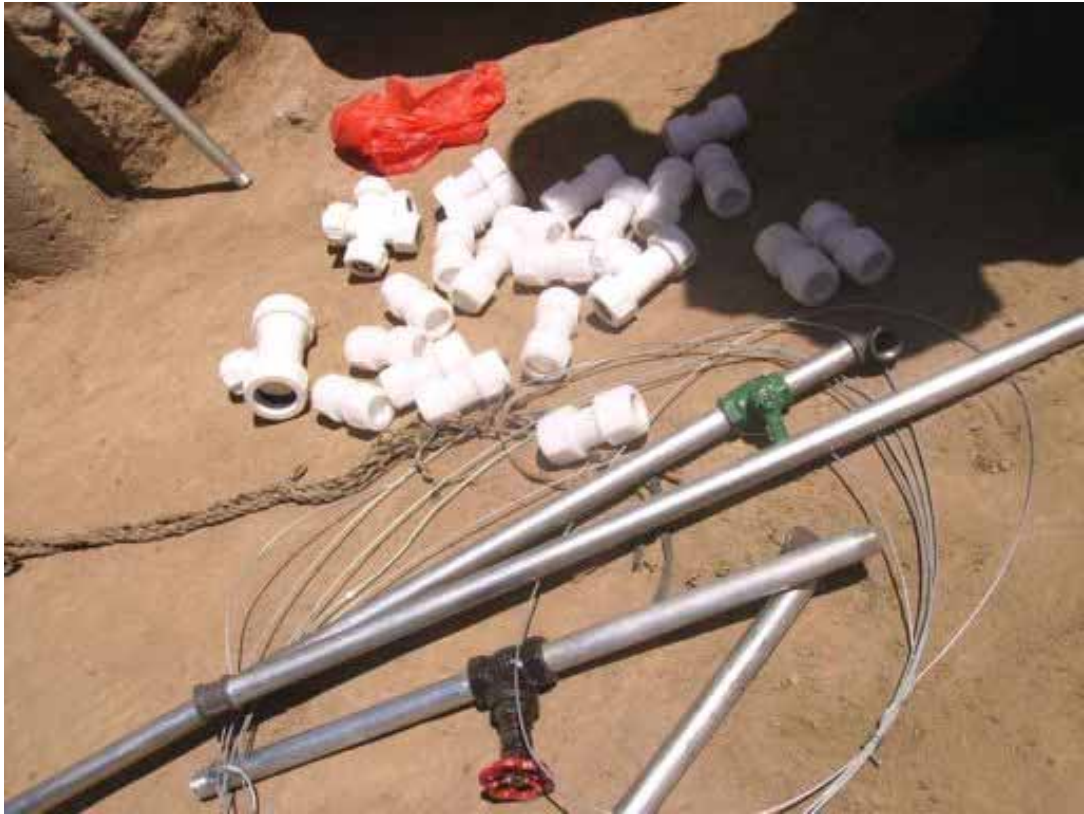
Pipe connections and iron pipes.
